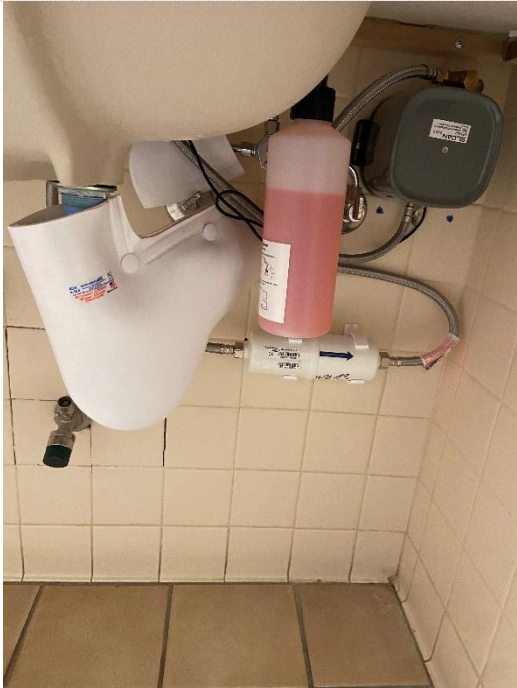
Photo #5: In-line filters installed 4.21.23 on bathroom sensor sinks
