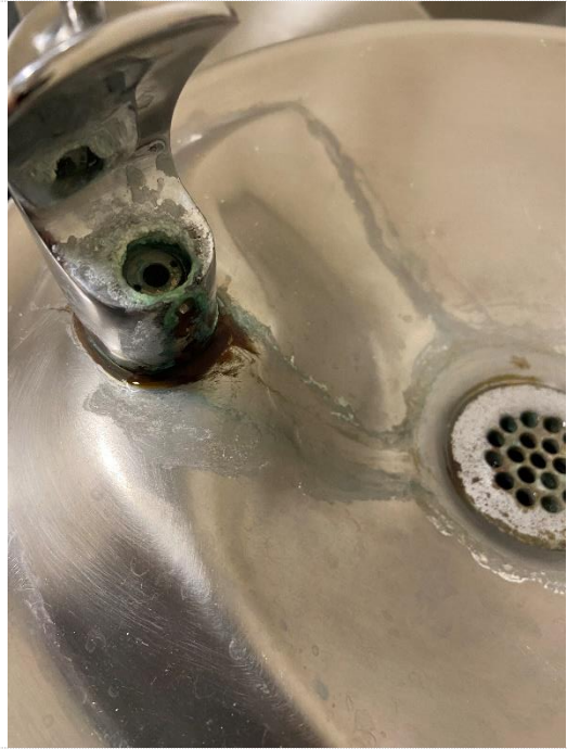
Photo #2: Evidence of scale on drinking fountain bubbler (Level 1)
