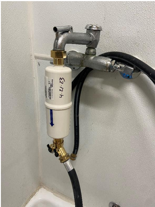
Photo #3: Janitor Closet Mope Sink – POU filters installed 4.21.23
