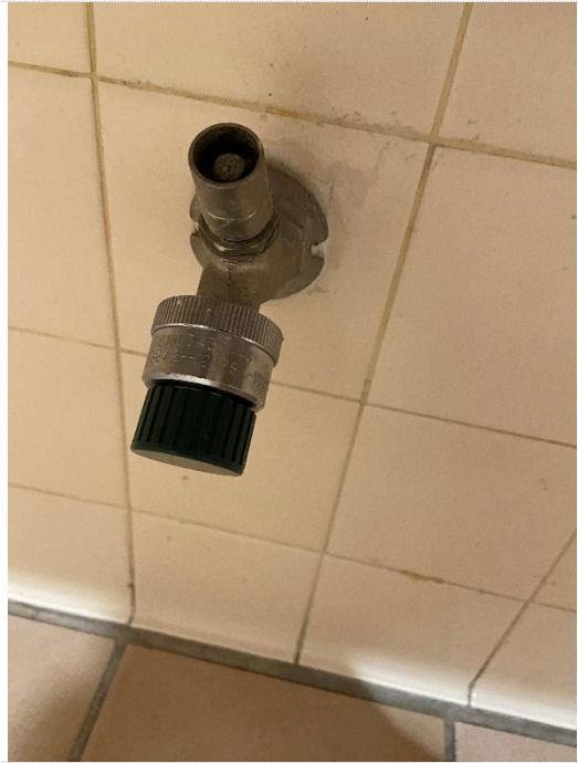
Photo #10: Hose bib under sink – Womens RR 24
