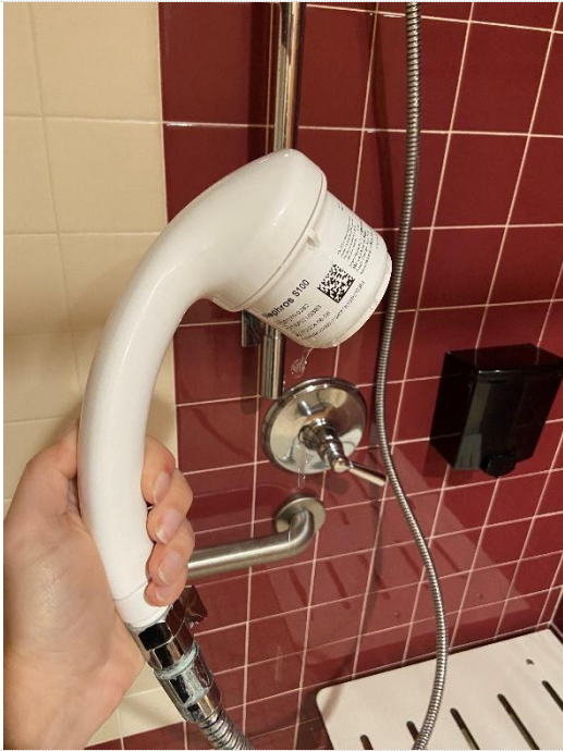
Photo #9: 1 st Floor – Shower – POU filter installed 4.21.23
