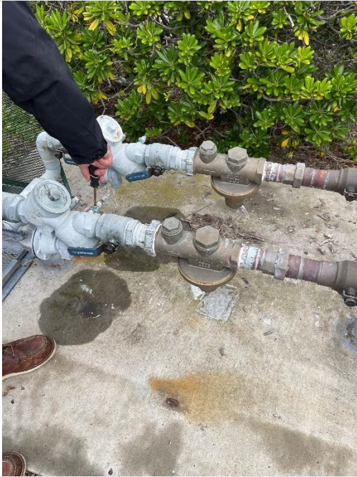
Photo #1: Municipal water connection
