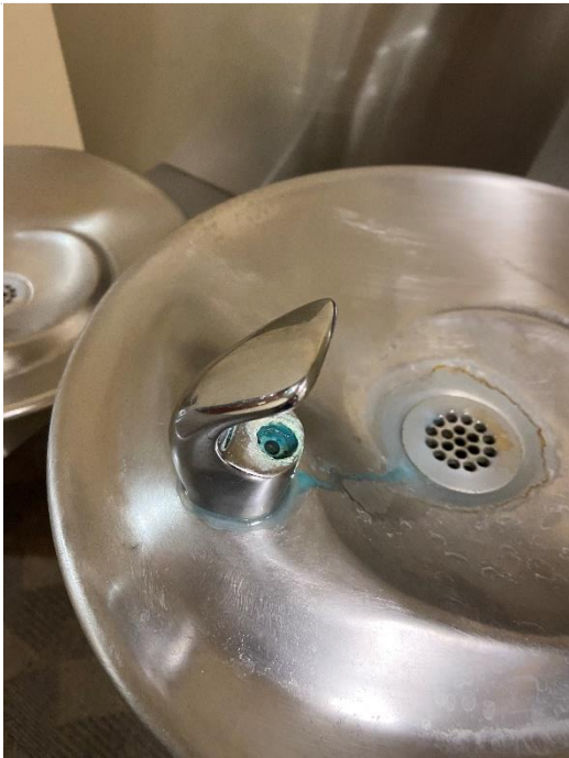
Photo #13: Evidence of scale on drinking fountain bubbler (Level 3)
