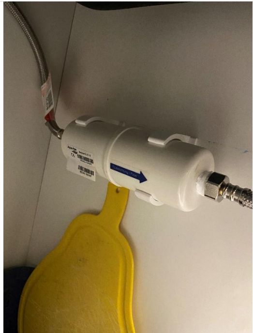
Photo #12: Inline filters under Ste 208 sink
