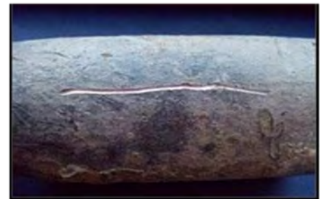
Picture of a Scratch on a Lead Service Line
