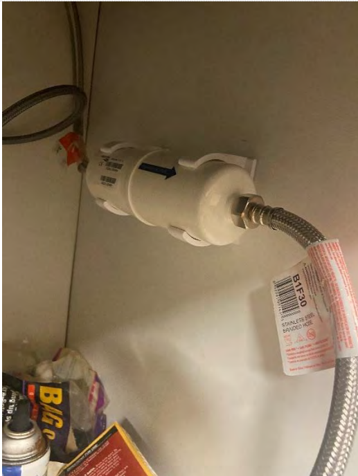
Photo #9: In-line filter installed under breakroom sink
