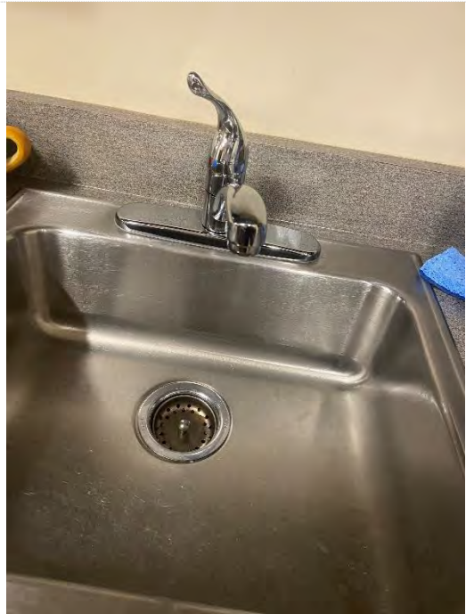
Photo #8: Mixer tap in breakroom
