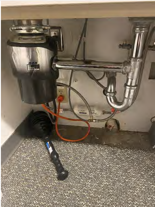
Photo #3: In-line filter - Suite 108 breakroom sink
