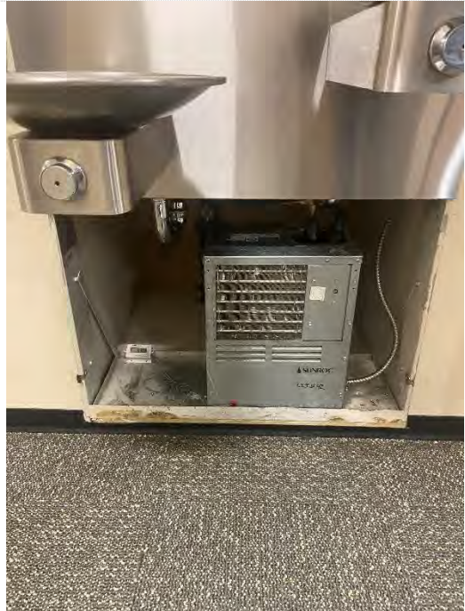
Photo #2: Cooler for water fountain
