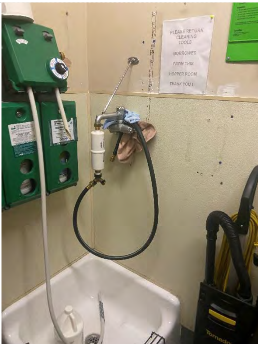
Photo #11: Janitor close sink – POU filter
