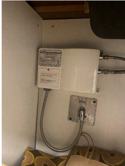
Photo #10: Water heater under breakroom sink
