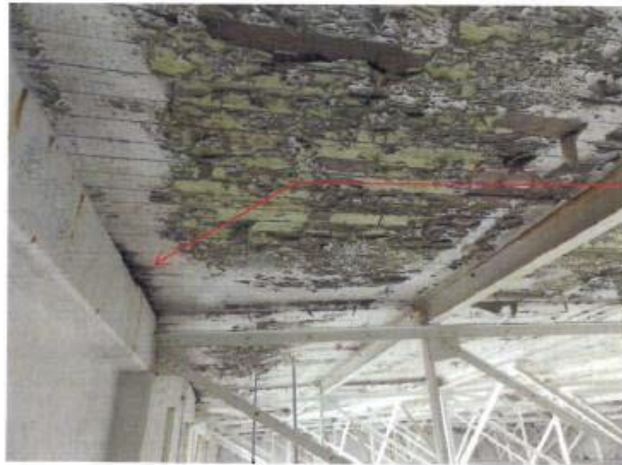
Structural Deficiency Due to Dry Rot
