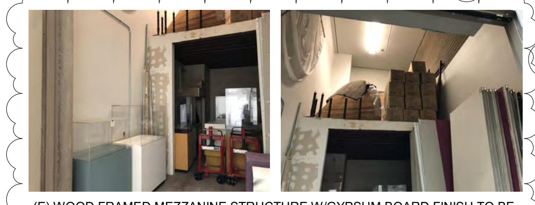
(E) WOOD FRAMED MEZZANINE STRUCTURE W/GYPSUM BOARD FINISH TO BE REMOVED IN STORAGE ROOM 164 PER KEYNOTE 2035
