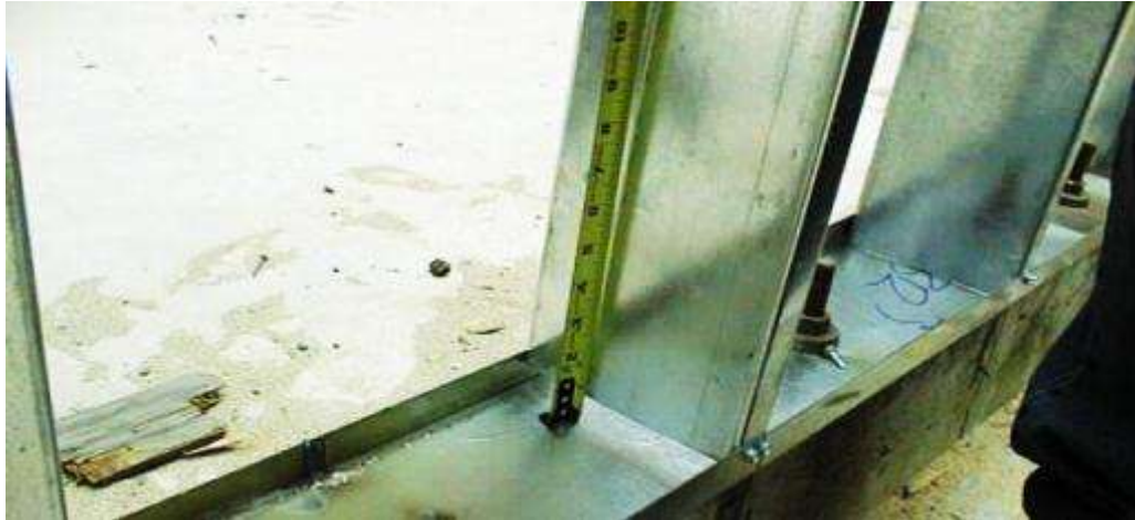
Figure 2-48: Incorrect Gap for Stud Bearing
