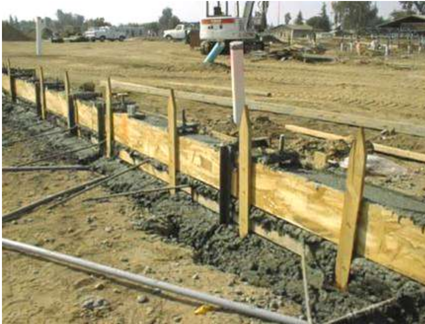
Figure 2-12: Lack of Tight Formwork; Wood Stake in Concrete Problems
