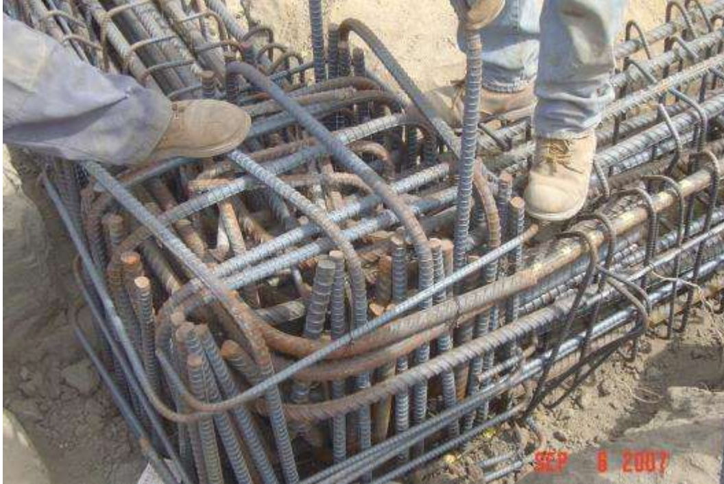
Figure 2-14: Extreme Reinforcing Congestion
