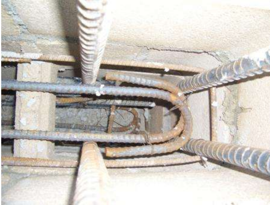
Figure 2-24: Congested Reinforcing in Masonry
