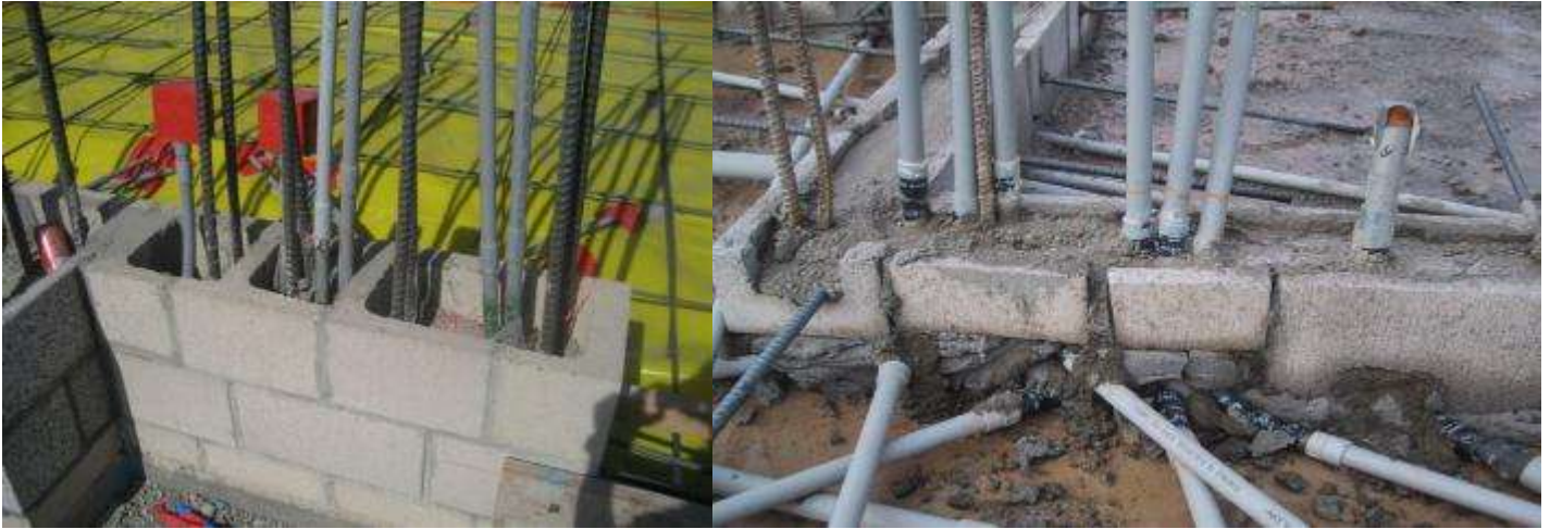
Figure 2-19: Coordination Problems in Masonry for Conduits/Pipes
