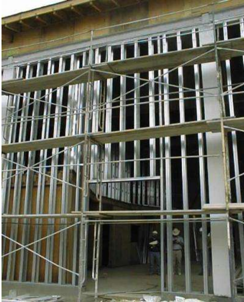
Figure 2-47: Single Jamb Supporting Header Insufficient - Multi-Stud Jamb Incorrect Location
