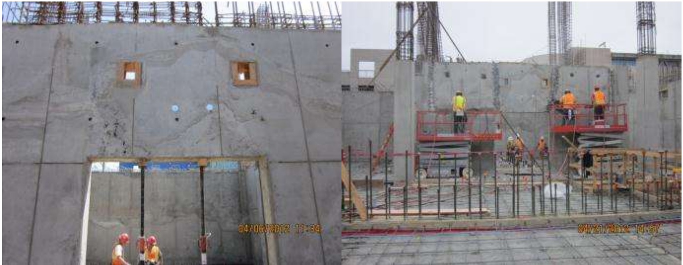
Figure 2-16: Poor Consolidation & Ensuing Repairs
