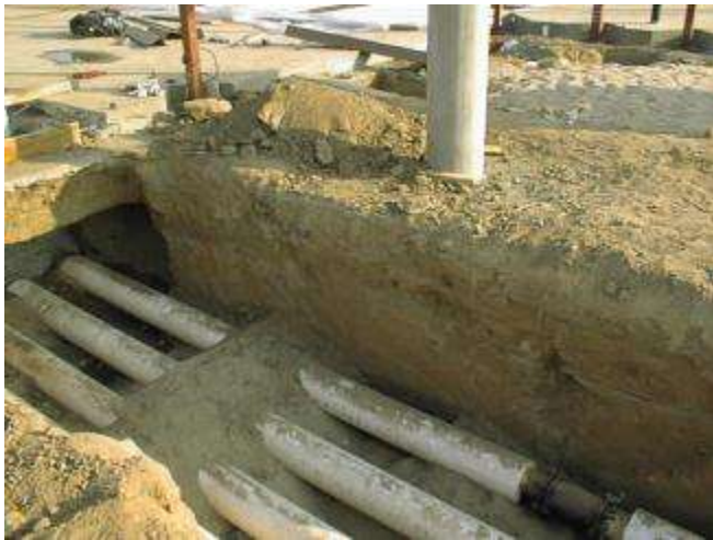
Figure 2-3: Improper Trench Location Due To Column Footing Proximity
