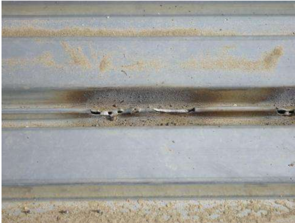
Figure 2-49: Additional Top Seam Weld Due To Burn-Through
