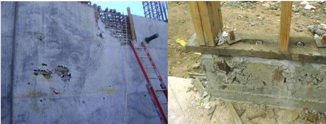
Figure 2-15: Poor Consolidation and Honeycomb Problems
