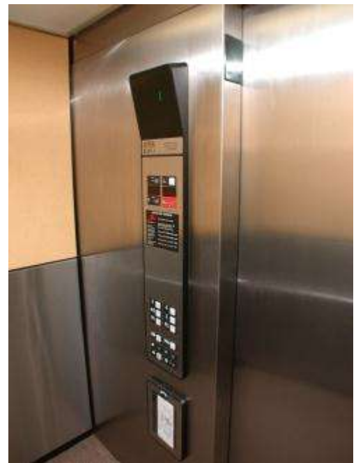
Figure 4-8: Elevator In-Car Controls
