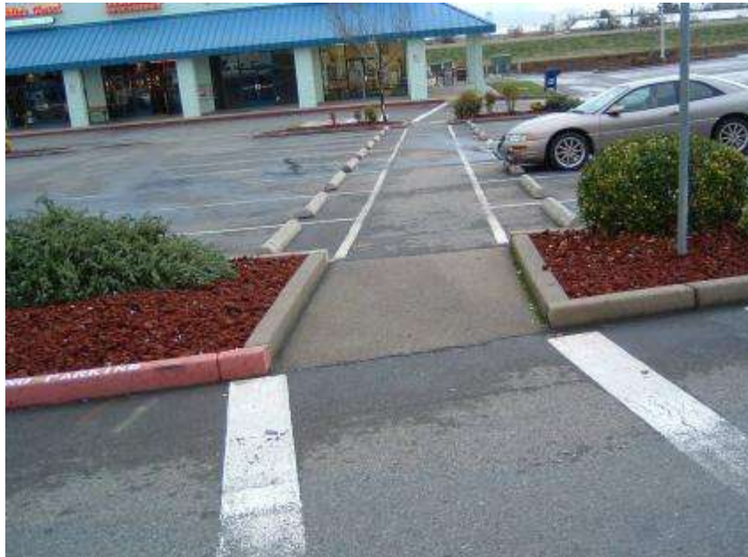
Figure 4-1: Path Of Travel at Site – Missing Items
