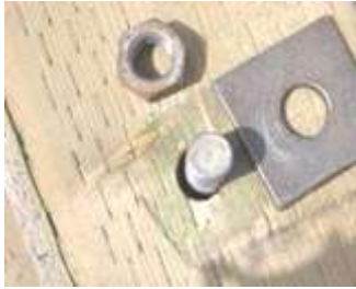
Figure 2-37: Improper Oversized A.B. Hole
