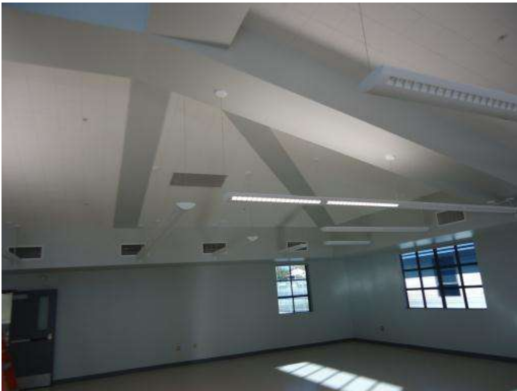
Figure 2-62: Pendant Lights Missing Safety Cables
