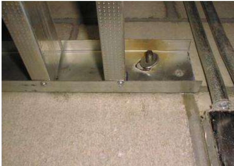
Figure 2-45: Oversized Torch Cut Hole
