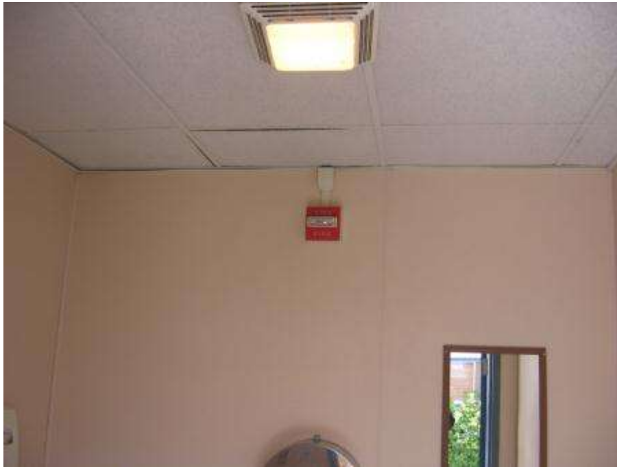
Figure 4-13: Example of Visual Fire Alarm
