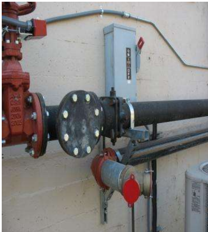
Figure 5-1: Improper Piping Location at AC Switch
