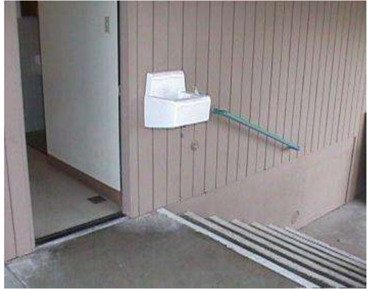
Figure 4-10: "Convenience" Drinking Fountain Causing Accessibility Violations
