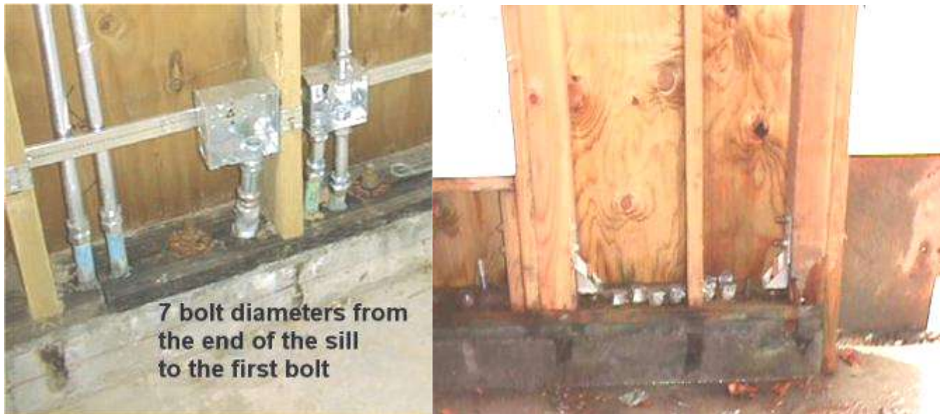
Figure 2-13: Common Conduit and Anchor Bolt Problems
