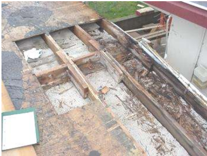
Figure 2-66: Water Damage to Roof Framing
