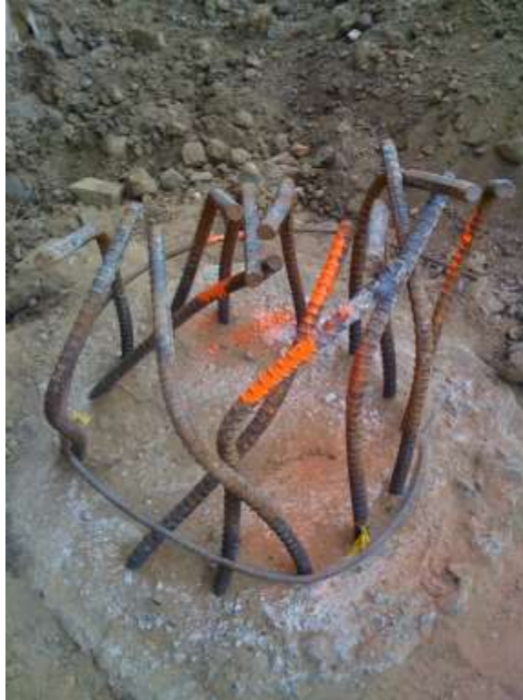
Figure 2-7: Damaged Reinforcement From Grading Operations
