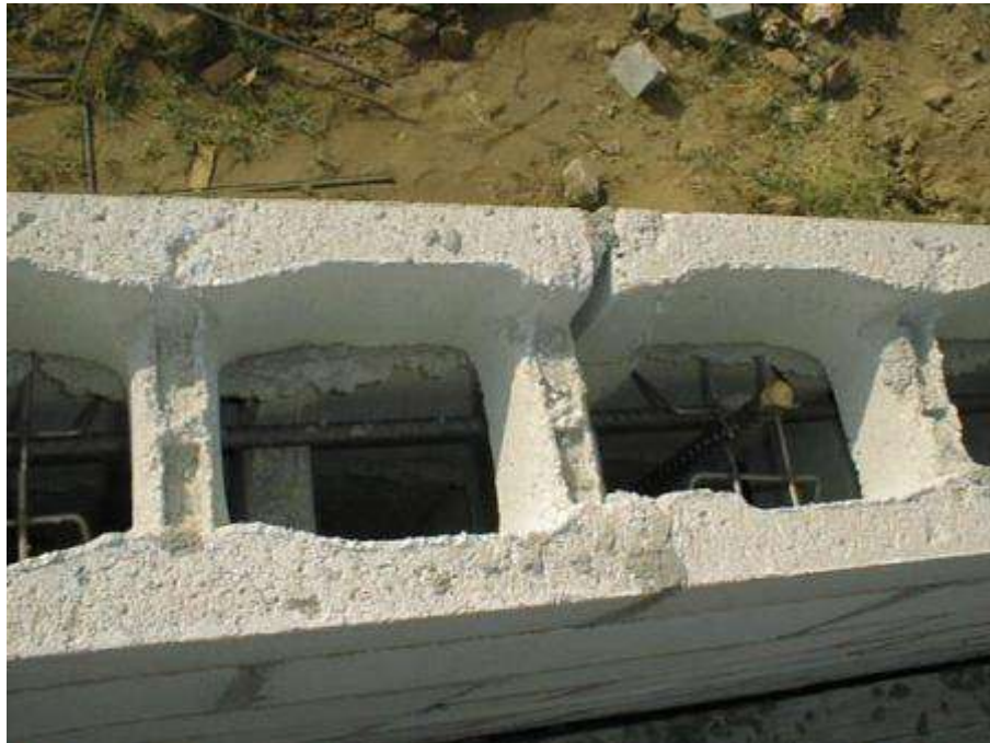
Figure 2-22: Lacking Full Head Joint; Mortar Fins Excessive
