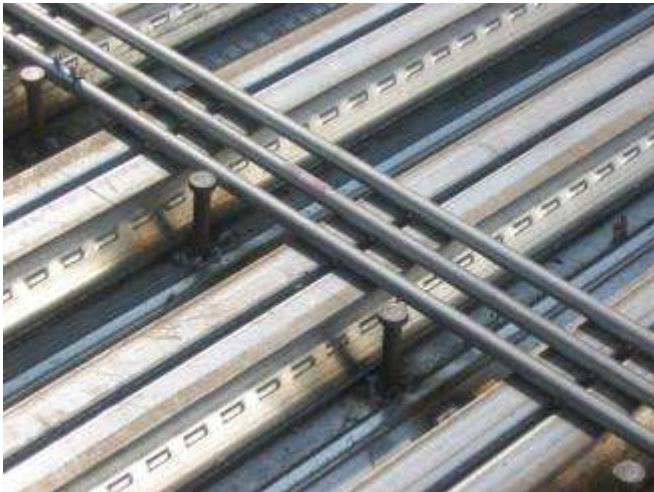
Figure 2-53: Conduit Causes Problems for Composite Action
