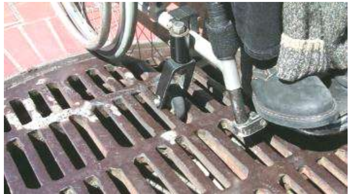
Figure 4-3: Incorrect Grating Type
