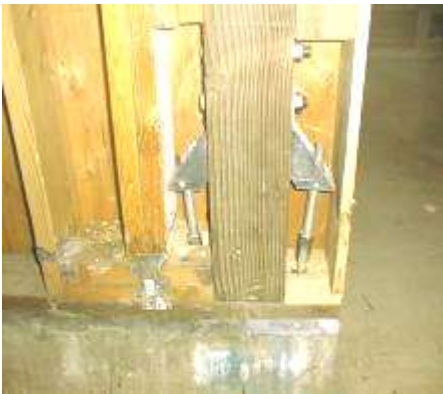
Figure 2-57: Hold-Down Construction Problems
